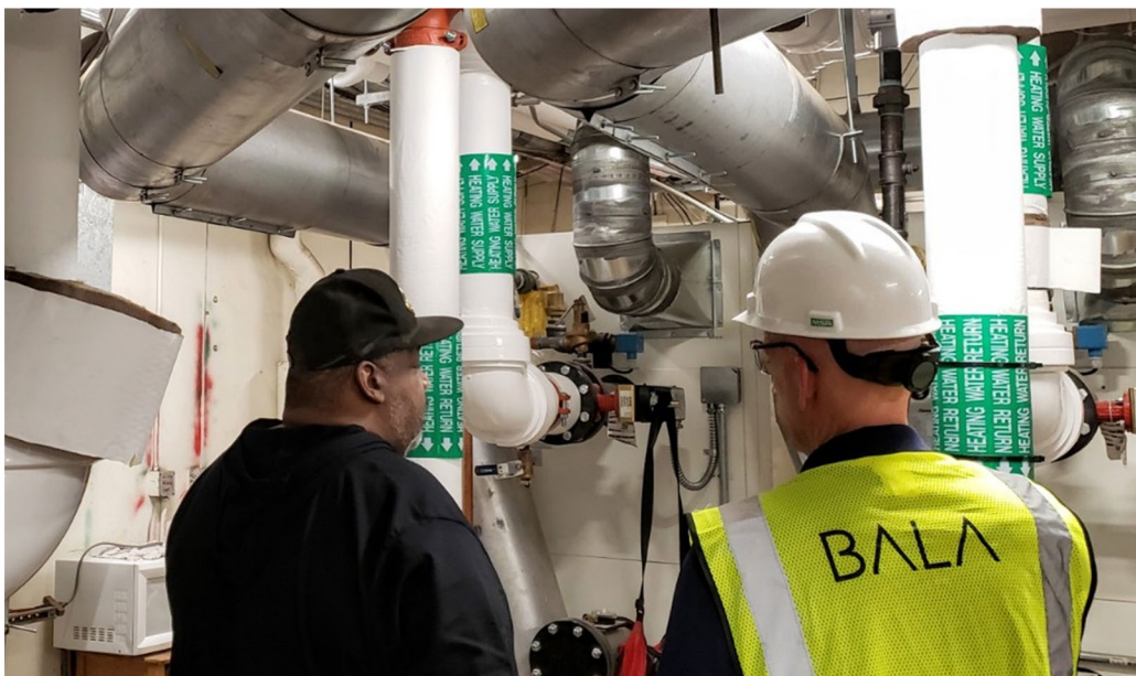
BALA Consulting Engineers reviewing the new chiller system and compressors at National City Christian Church Washington, DC
